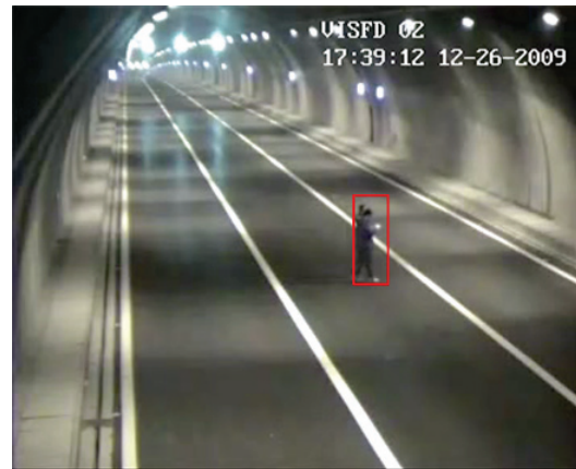
Figure 3. AlarmEye VID system for security protection in a road tunnel
