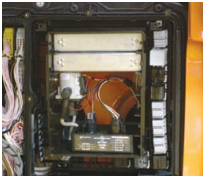
Left: Battery Guard 3,000 will ensure a full battery for fire appliances. Above: Battery Guard enables different parameters to be recorded into it.
